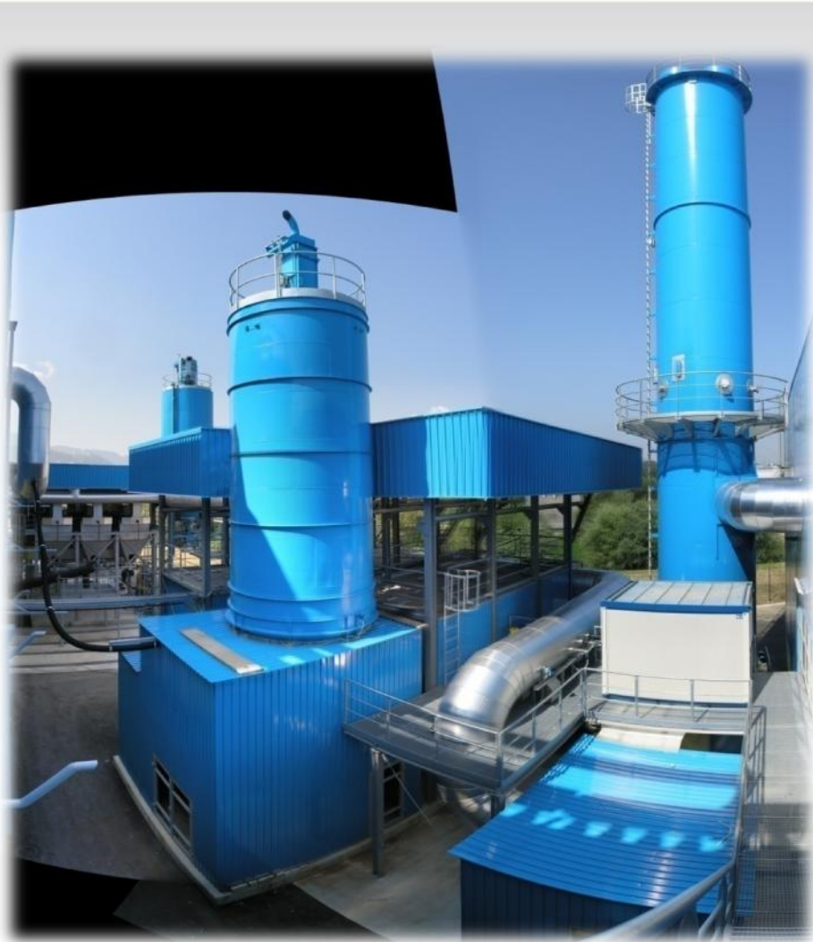
Activated carbon filter, CEMS and stack
