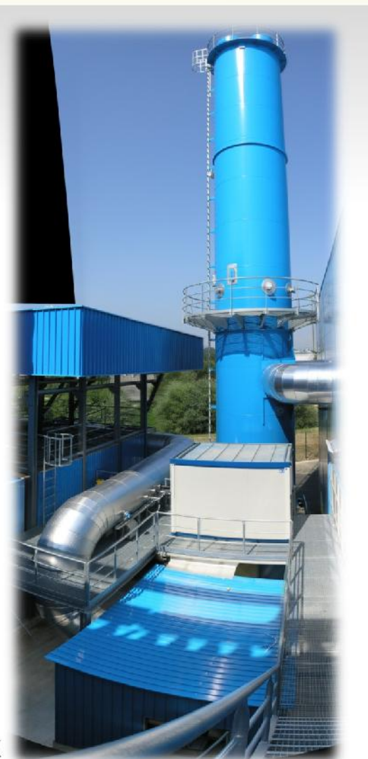
CEMS and stack
