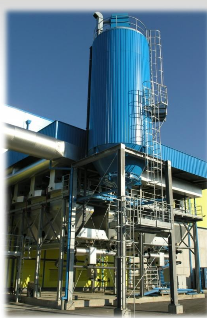
Ceramic filter and fly ash silo
